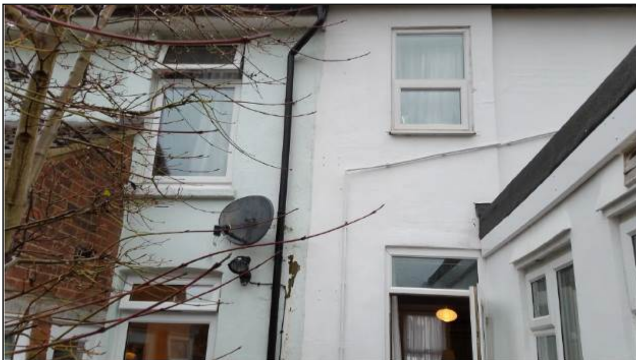
Figure 8 - rear of No 42 (white) & No 44 (pale blue) – affected bedroom window above satellite dish
